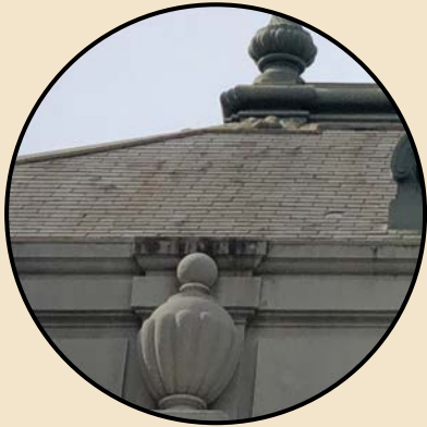
Inappropriate building material
